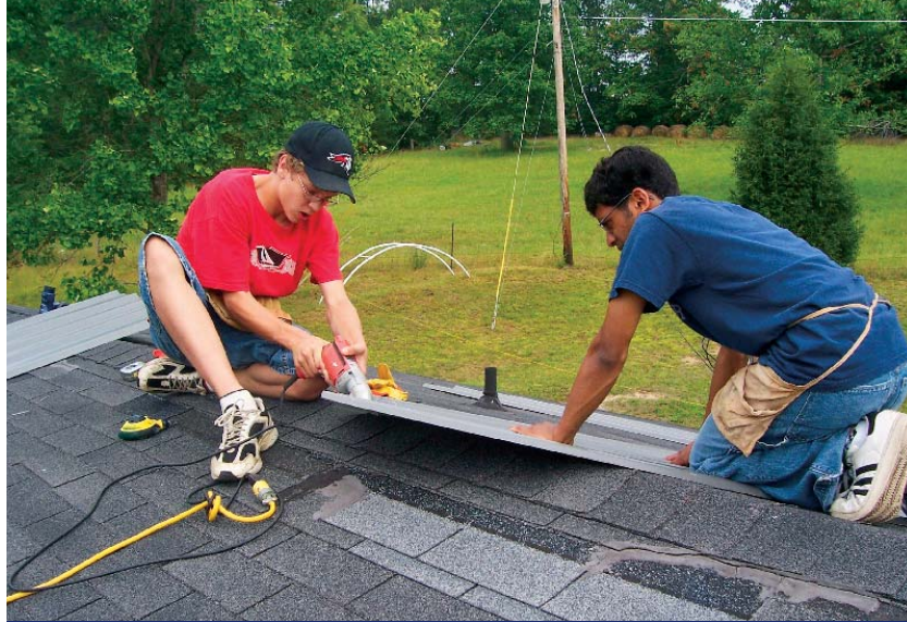
Thomas and Mark, two volunteers from Columbus (Ohio) Mennonite Church, put down a metal roof for a homeowner in Eolia, Kentucky.
